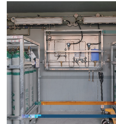
Mixed Gas Supply Station
